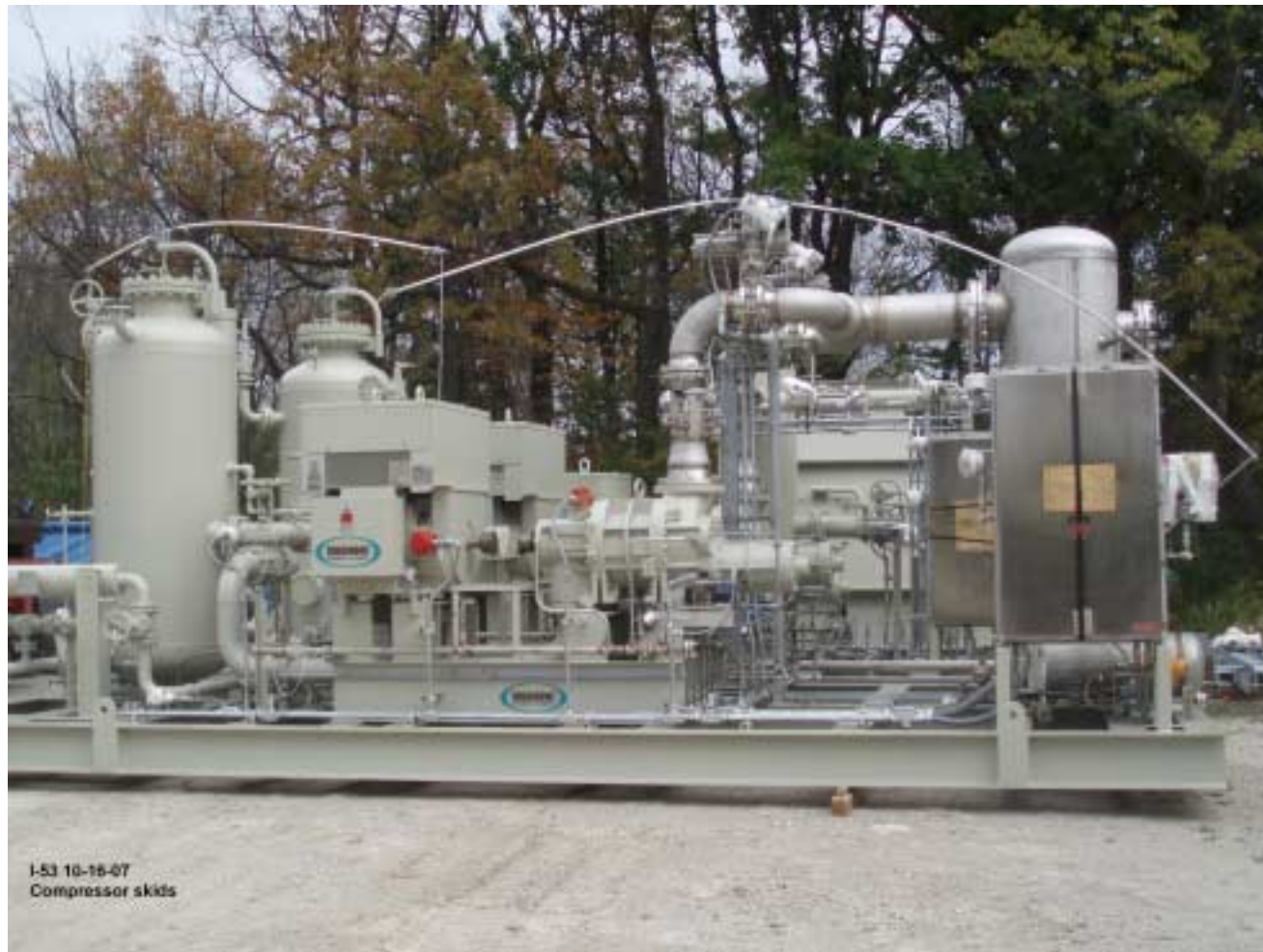
Gas Compressor Skid
