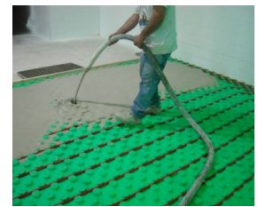
Radiant Floor Heater
