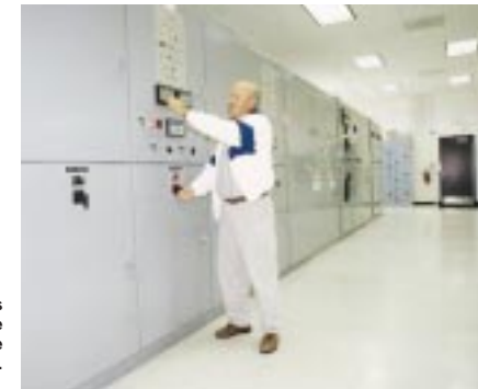
Jim Brown, Charles Equipment Co., monitors the generator controls in the Zoo's cogeneration plant.
